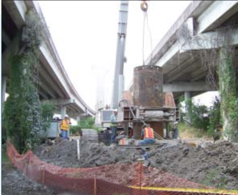
Even the areas with no overhead obstructions were tight to access and difficult to maneuver through because of the existing structures and foundations.
