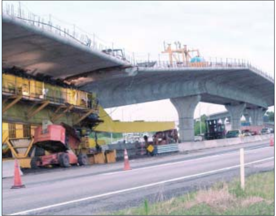
Foundation failure at Bent 97 - April 13, 2004. Photo courtesy of PCL Civil Constructors.
