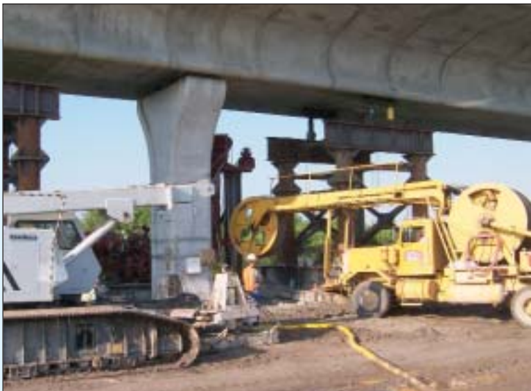
BECK designed and built concrete pump placing concrete into shafts with overhead restrictions.
