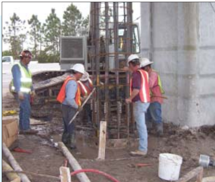
Rebar cage consisting of (12) #18 vertical bars being spliced together with mechanical couplers.
